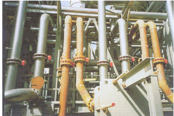
Photograph 3 : Composite Material Piping in an Offshore Platform
