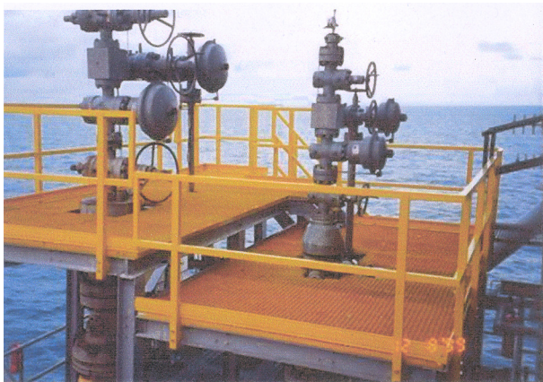
Photograph 2 : Composite Material Grating and Handrail in Offshore Platform in Well Head Area
