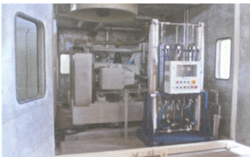
Fig.4 Burckhardt Compressor with Driers
