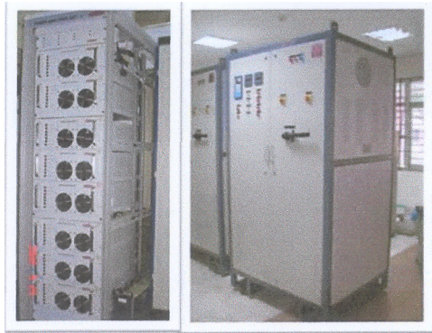
Fig.13 Power Amplifier Rack with Power Supply
