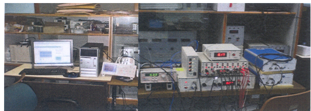
Fig.10 Control System Electrics for ASAC
